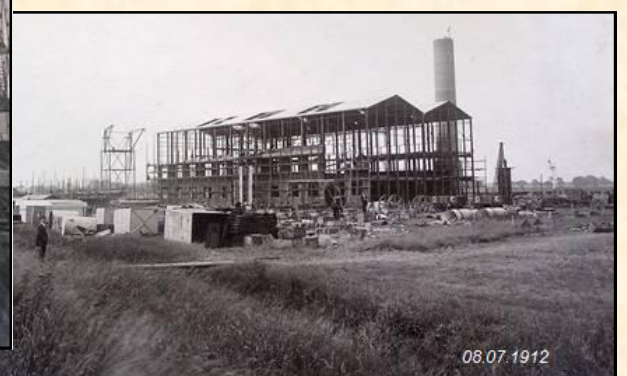
Photos left and below: Framework almost complete and boiler chimney built 1912 © British Sugar PLC, Cantley
